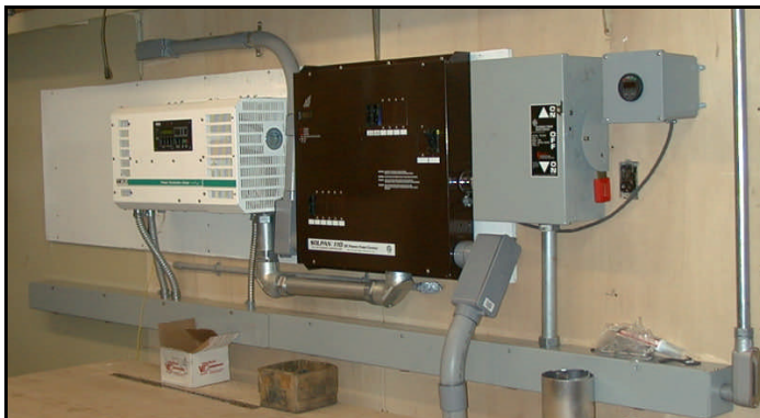
Inverter, Charge Controller/Circuit Breakers, and Transfer Switch
